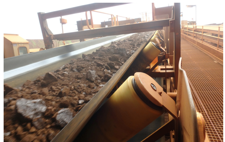
The ECS project demonstrated an integrated approach between client and OEM to successfully remove unnecessary conveyor downtime
